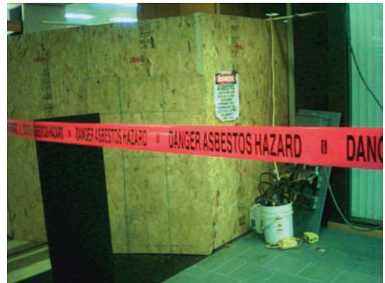
An area in an office building undergoing the removal of asbestos, a hazardous air pollutant. (Aaron Suggs/Creative Commons)
